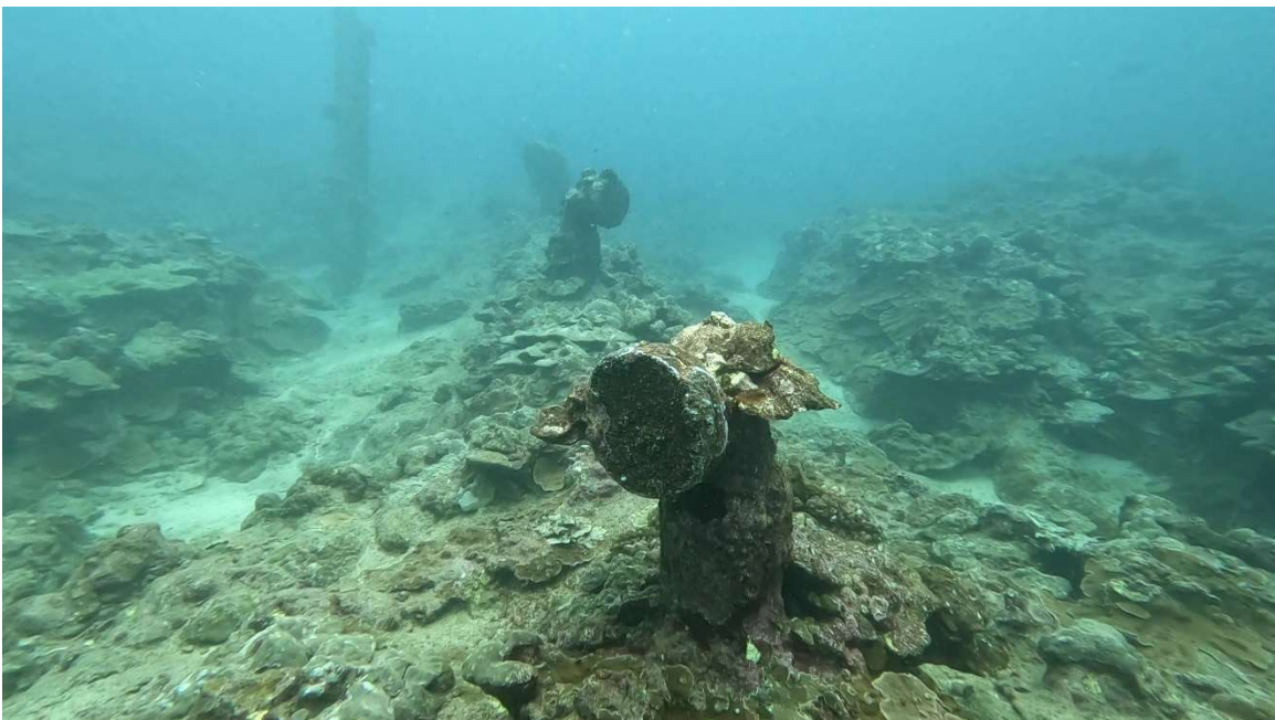
Figure 18. Typical view of original diffuser ports and riser landward of manhole #2 with blanked port flanges visible
