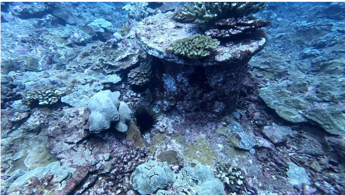
Figure 12. Manhole #A2 located at Station 39+78 with coral cover but visible outfall pipe
