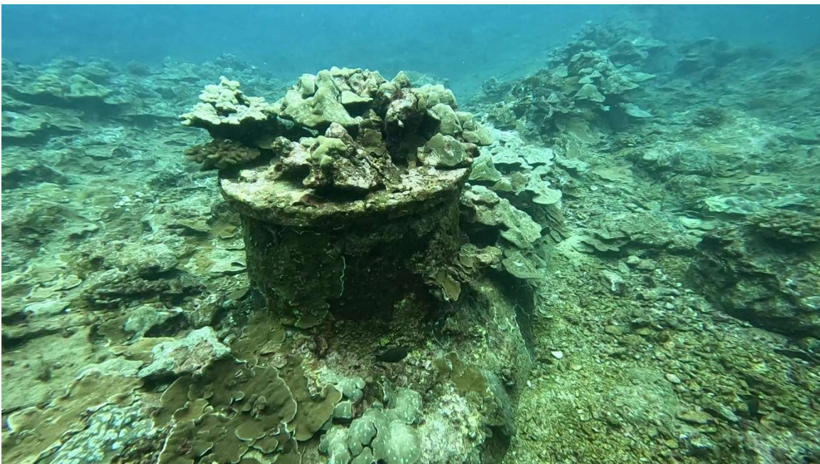
Figure 10. Manhole #A3 located at Station 42+23, with extensive coral cover but visible outfall pipe
