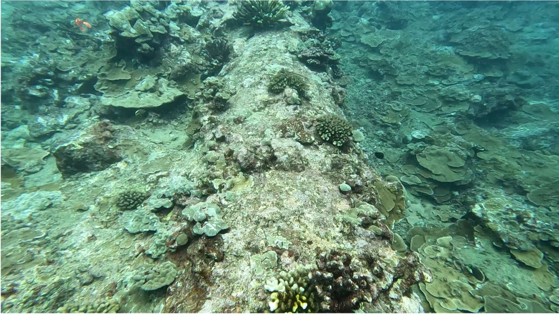
Figure 13. Section of outfall with scour on one side near Station 39+15
