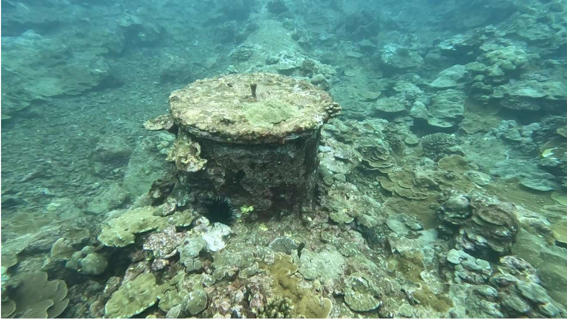
Figure 15. Manhole #A1 located at Station 30+95 with coral cover but visible outfall pipe
