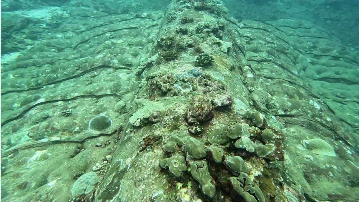
Figure 11. Outfall pipe with concrete mattress repairs performed in 2016, Stationing 41+92 to 41+54
