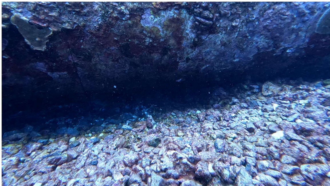
Figure 14. Section of outfall found with scour on both sides, vicinity of Station 33+15
